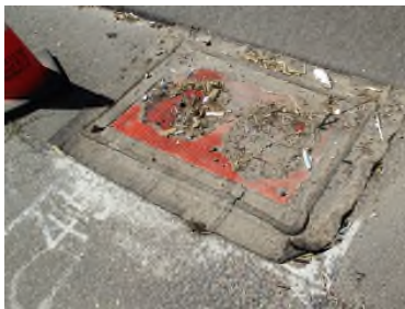
Year 2: Post storm—before cleaning
