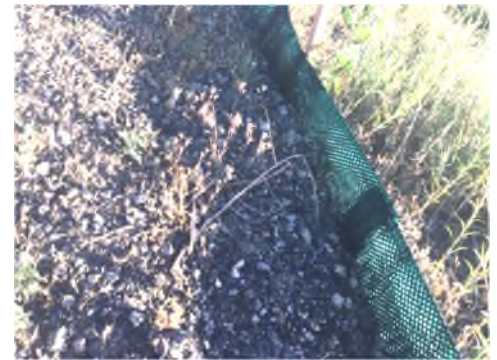
By springtime, 100% of ProWattle was functional and continued to perform until project completion.
