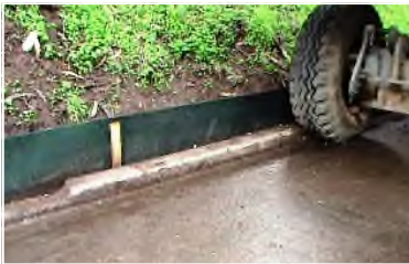
S-Fence™ - protection at base of slope
