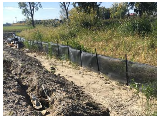
E-Fence with Sediment Control Panel Sediment capture post storm
