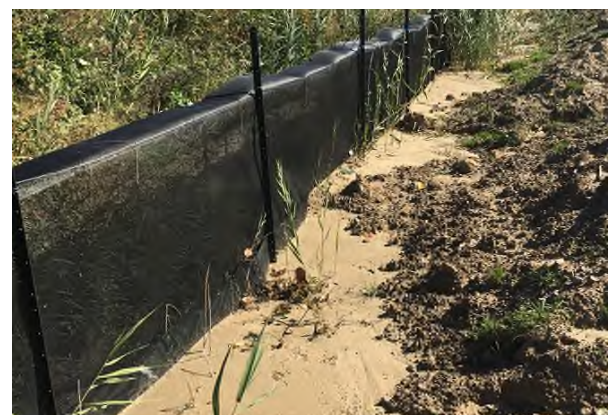
E-Fence with sediment control in the same trench, eliminating the need for a separate silt fence or wattle
